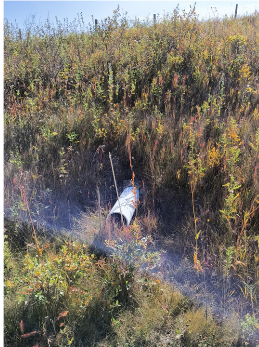
Figure 10 Wastewater Lagoon Release Pipe
